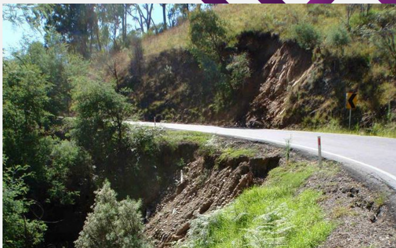
Landslip on the Bogong High Plains Road
